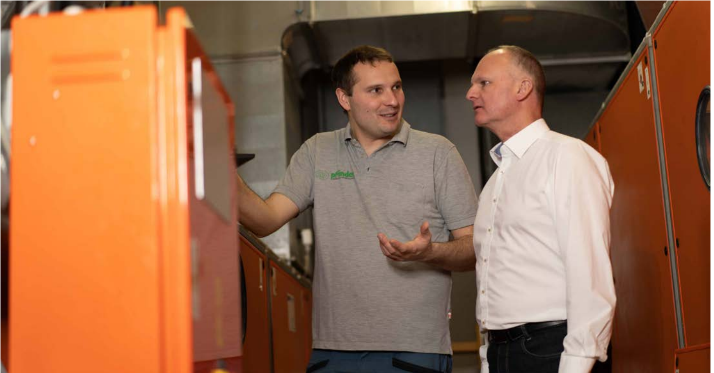
FIGURE 1: Lukas Pfänder, Managing Director Pfänder GmbH and Ralf Braun, Sales Director Germany, inspect the ventilation system in Beutelsbach monastery cellar.
